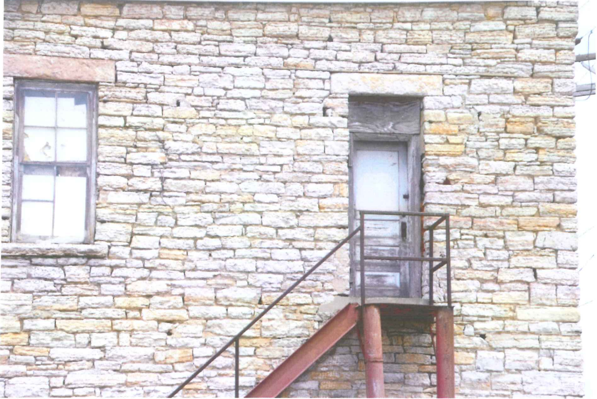
Detail of the fire escape stair on the rear façade. Note the original window and condition of the stone.
