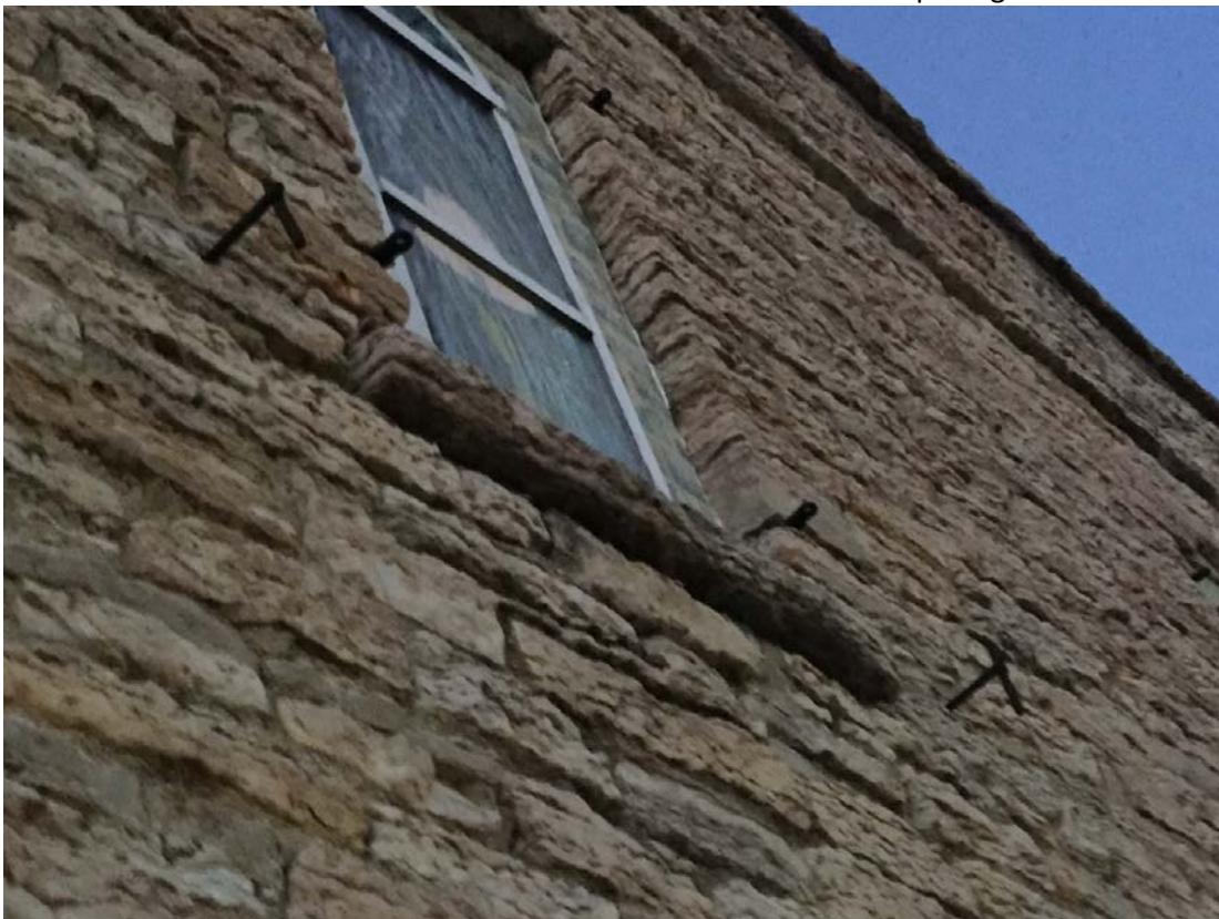
Detail of metal tie rods on the south façade (south façade only).
